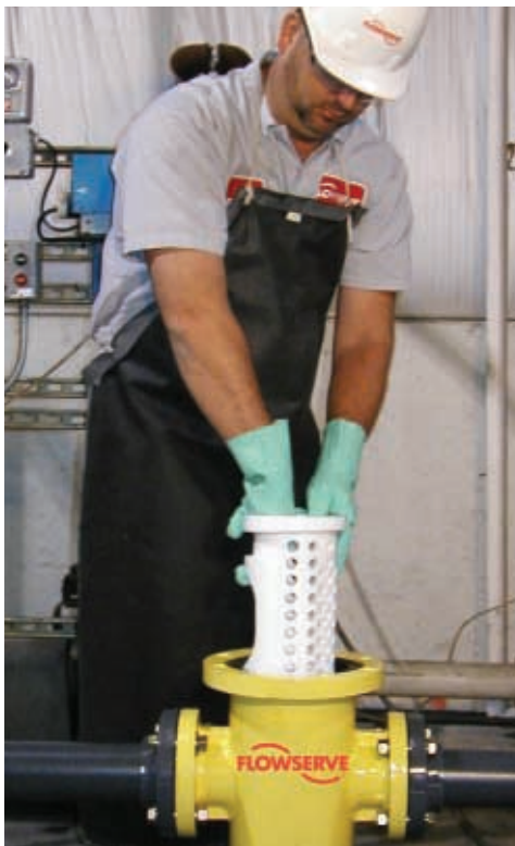
Removal of basket
